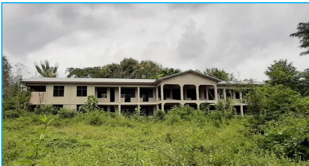
Pic. G. 2 story community health nursing training hostel at Asafo (Sefwi Wiaswo Municipal Assembly)
